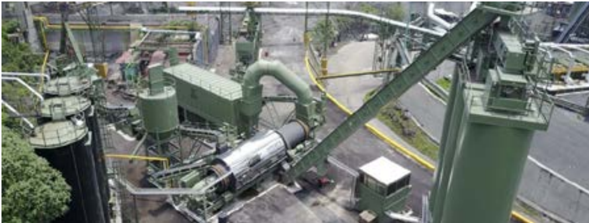
Figure 18. Asphalt plant are continuously evolving to capture emissions from being released to the atmosphere. Image from World Highways website.
